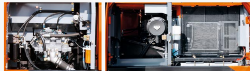
Grouped remote filters and inspection points
